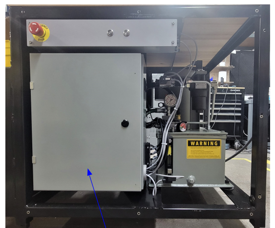
Front of Cabinet (cover removed)
