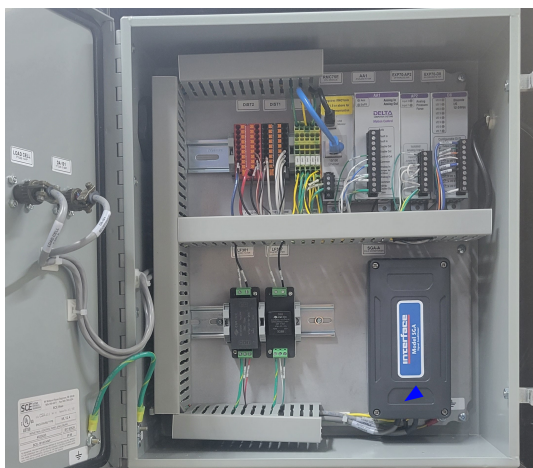
Delta Controller Enclosure
